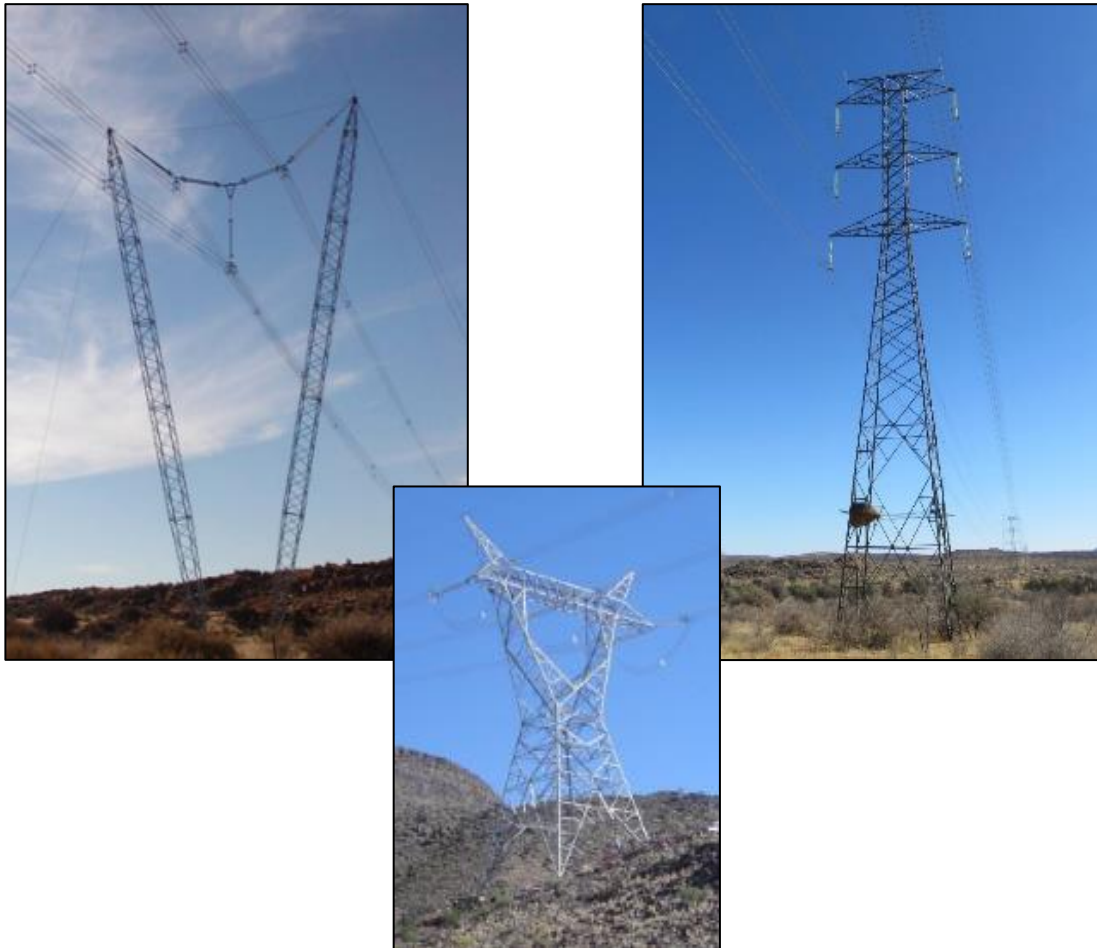
Figure 2. The structure of the pylons for the planned 400 kV power line, showing the V-type guyed (cross rope) suspension tower (used for 90% of the line) (left), and the self-supporting strain structure (inset); and the self-supporting pylon of the existing 220 kV power line (right); the structure for the 220 kV strain towers is similar.
